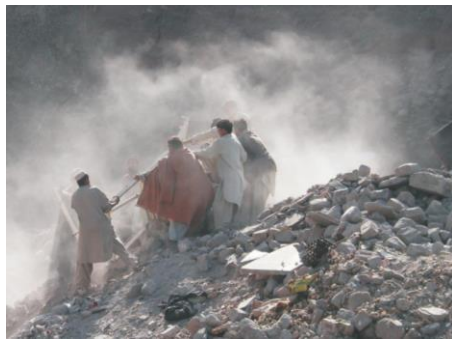
not work boots. They too lack any form of respiratory or eye protection. In both cases, these workers are subject to immediate risks simply associated with these types of activities but given the lack of respiratory and eye protection, they also could be subjected to risks associated with exposure to dust and organic volatiles (potentially containing asbestos and other carcinogens).
